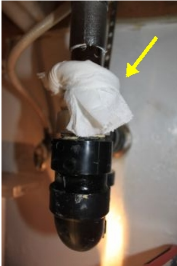
Drain line leaks under sink. Small leak at hall bathroom sink.
