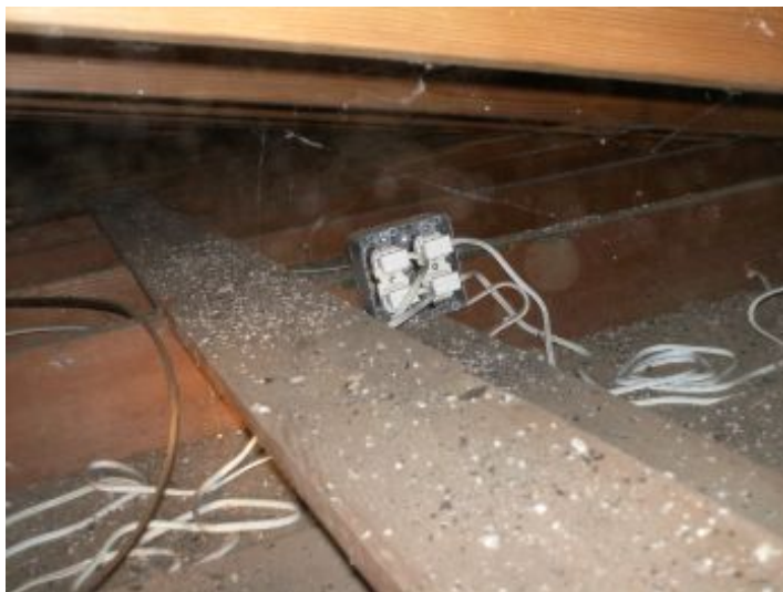
Open receptacles & non-standard wiring installation are present in the attic
