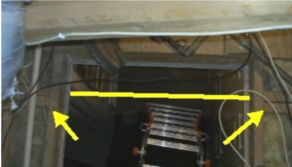
Roof truss bottom cord has been cut out. Alterations to trusses are not permitted without engineering.
