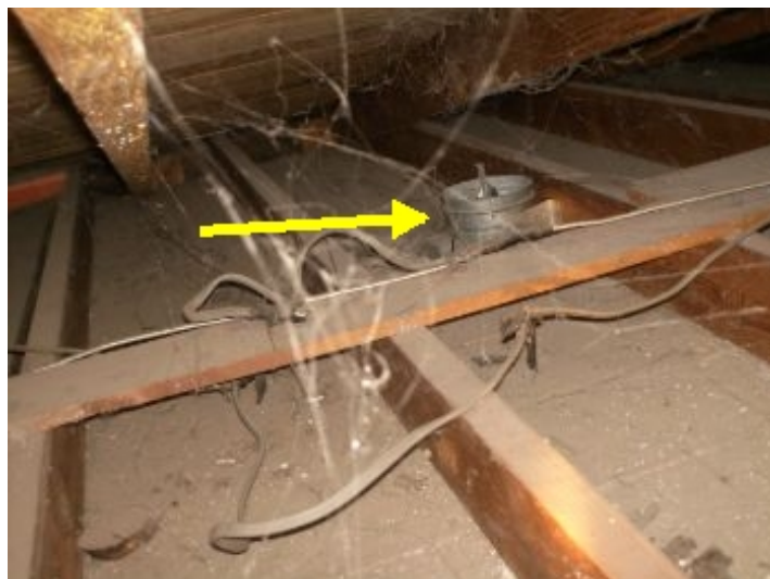
Bathroom vent terminates in attic rather than venting to exterior
