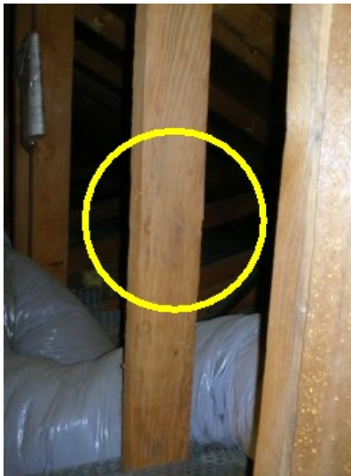
King post of truss is cracked. Repair recommended.
