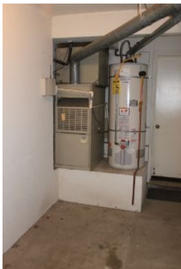
Water heaters in garages should be protected from vehicle impact
