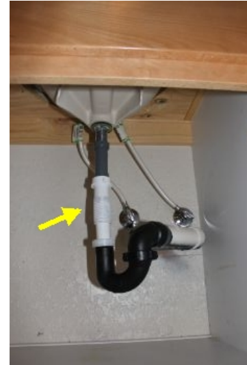
Flexible tubing is a non-standard material for this application
