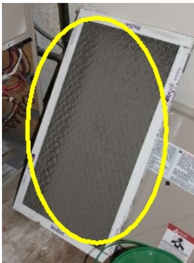
Air filter needs to be changed regularly
