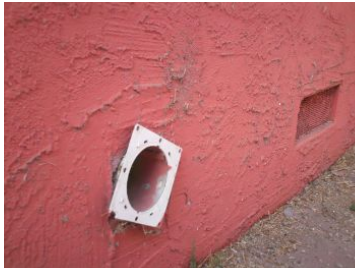
Dry vent missing screen and damper
