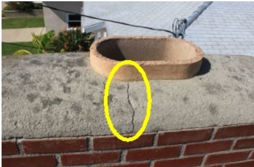
Crack in chimney crown should be sealed
