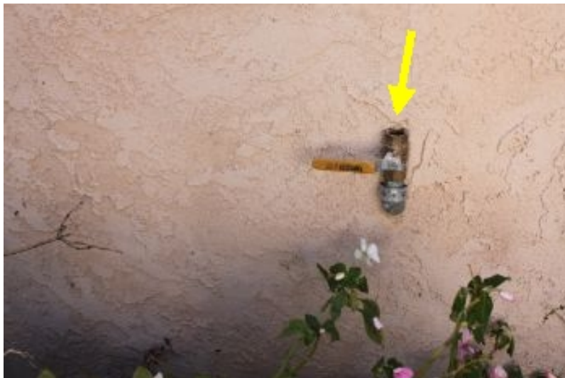
Uncapped gas valve presents a hazardous condition
