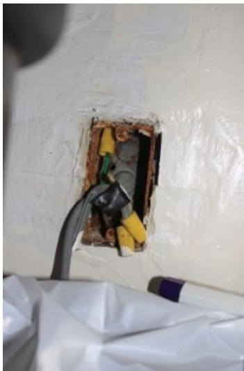
Junction box missing cover and wires are exposed.
