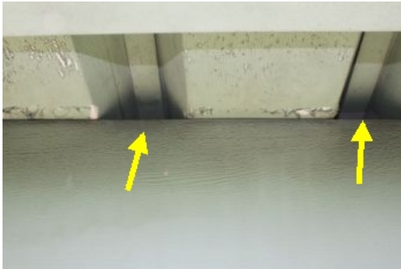
Some places are missing insulation / birdstop under sunroom roof.
