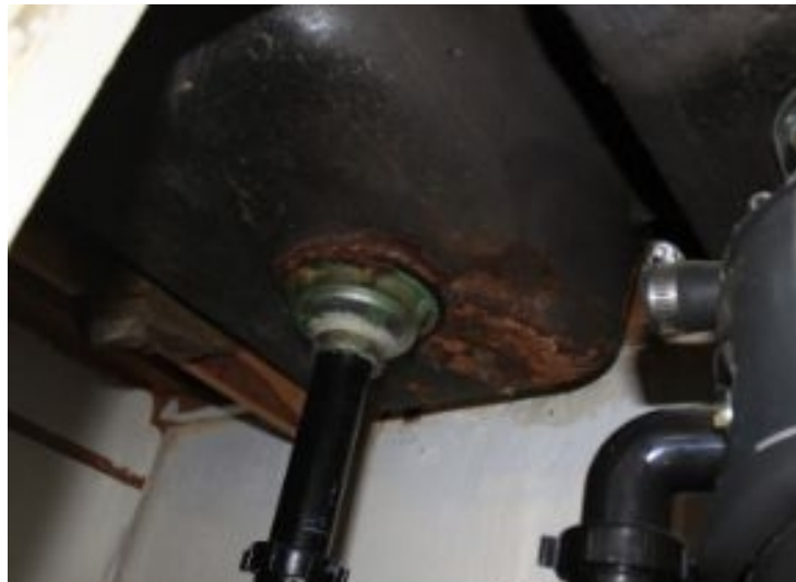
Rust at underside of sink
